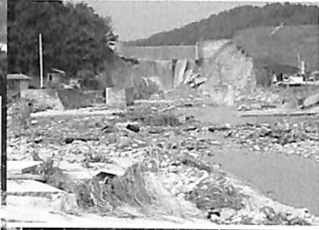
Gyungpo reservoir spillway was broken
